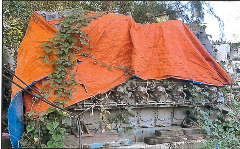
Port Main Engine Paxmen Valenta / 16RP 200M
